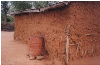
A simple roof catchment system with gutters
