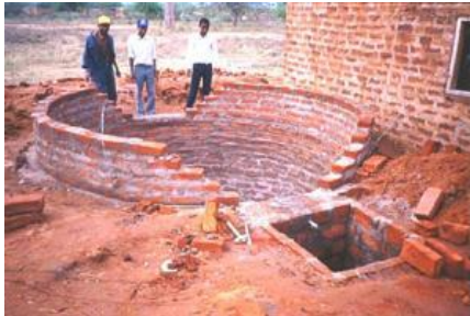
Cylindrical ground tank
