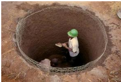
A cylindrical ground tank made of ferrocement
