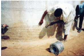
Chicken mesh and barbed wire wrapped around a cracked tank.
