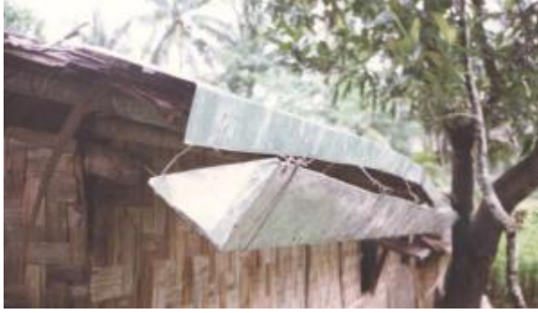
Gutters fitted into hangers tied to a splash-guard nailed onto an uneven roof
