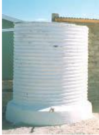
A repaired tank
